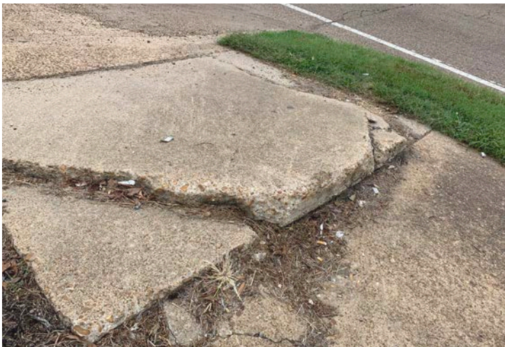
Pedestrian facilities (sidewalks in particular) are poorly maintained.
